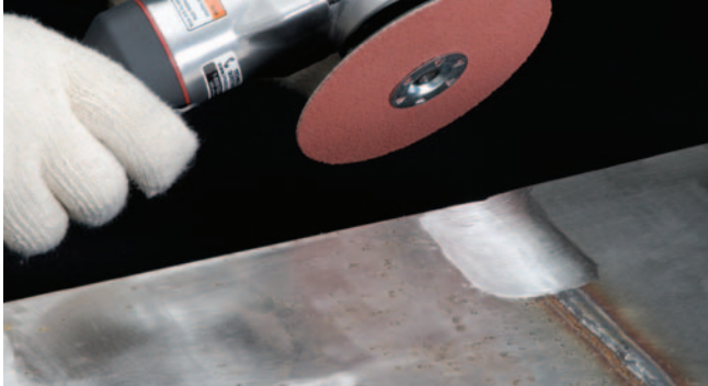
PRODUCT: 5" Pinnacle Resin Fiber Quick Change Disc, 36 grit APPLICATION: Weld removal on Stainless Steel table.
